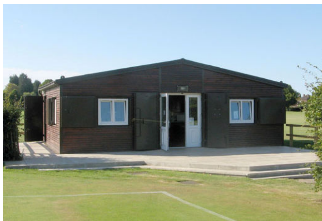
The Chester clubhouse, showing the heavy steel covers for the doors and windows.
